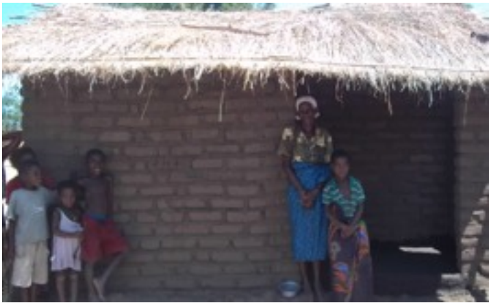
A new home constructed with the support of MCV in Bolera Village for a family that previously had no shelter
